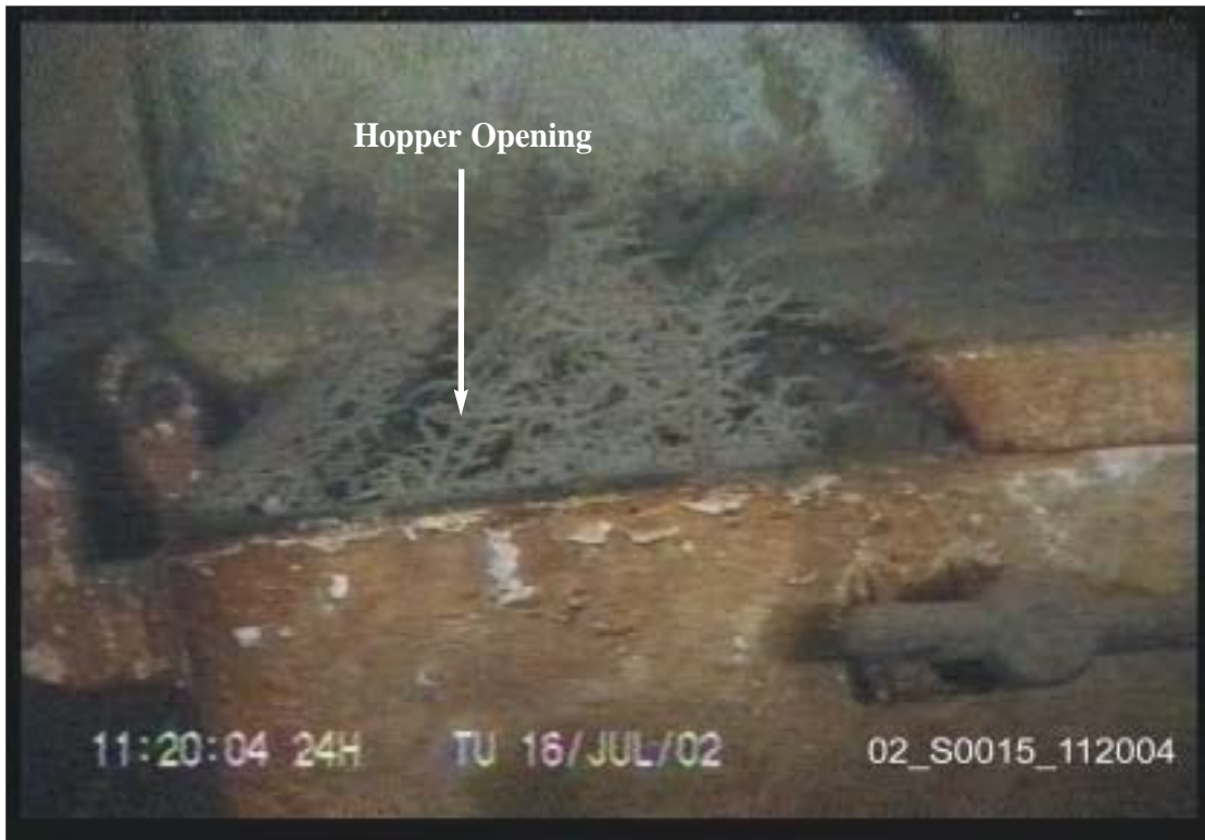
Offal Chute Split Covers (Chute C2)
