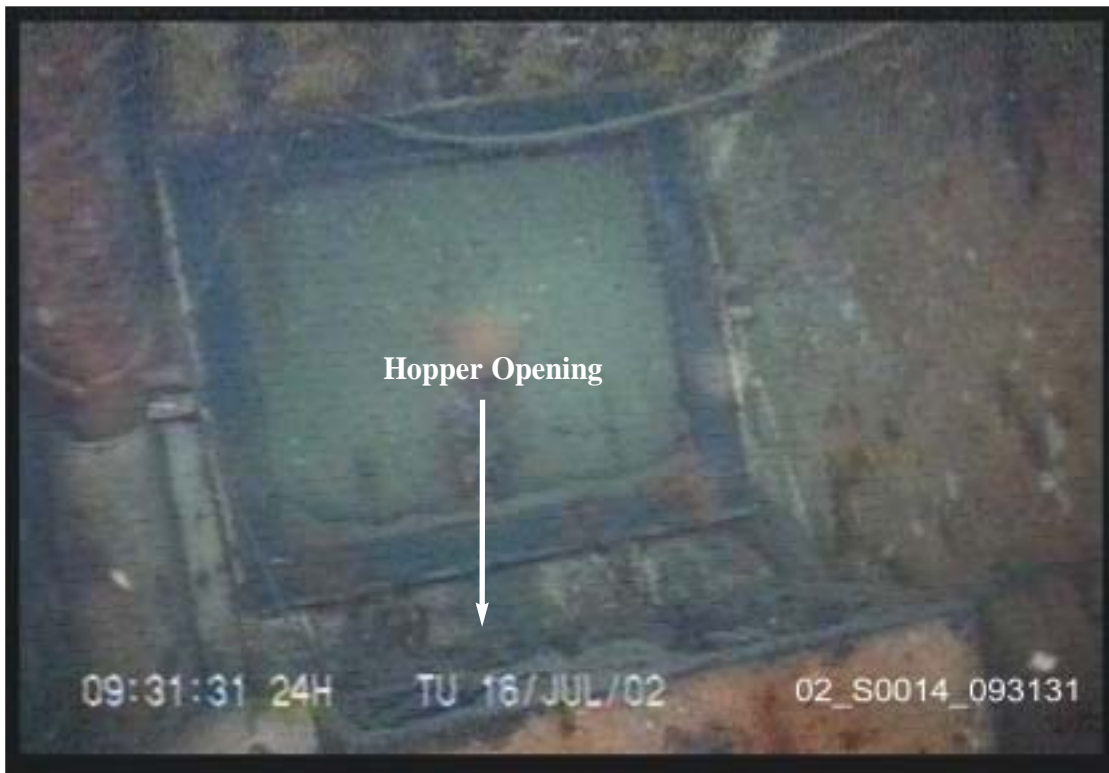
Duff Chute Cover (Chute C1)
